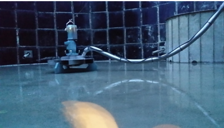
The OKI 2000 E-37AM with air hose at the bottom of a circular aeration tank.
