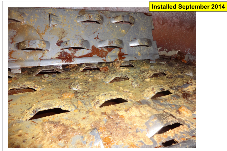
Figure 6 XVG trays in an ethanol plant's beer tower
